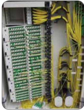
Poor Cable Routing
