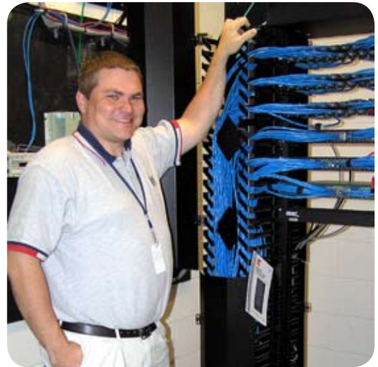
Steven Compton, director of IT at Franklin Road Academy, considered total cost of ownership and decided to implement ADC's 10-gigabit CopperTen copper cabling to last a minimum of 20 years.
