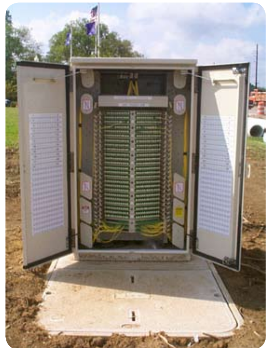
ADC's FDH 3000 Cross-Connect Cabinet effectively manages and protects EATEL's OSP fibers.
