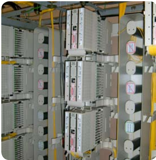
EATEL uses the NGF frame to terminate, route and protect fiber in their central offices.
