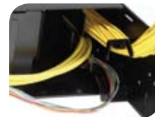
Proper cable management avoids fiber damage that can result in signal attenuation.
