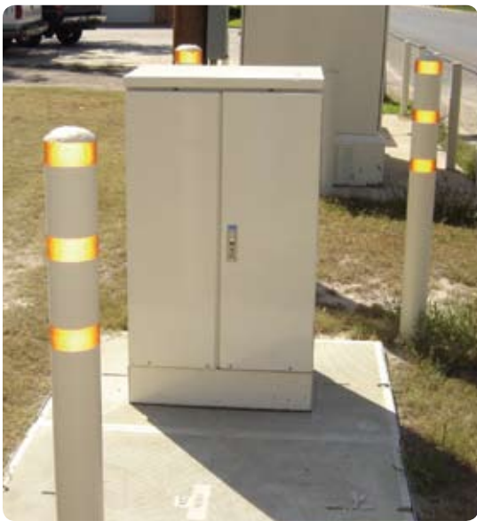
ADC's OmniReach® Fiber Distribution Hubs and Fiber Access Terminals proved rugged enough to handle the dry, dusty winds of northwest Texas.
