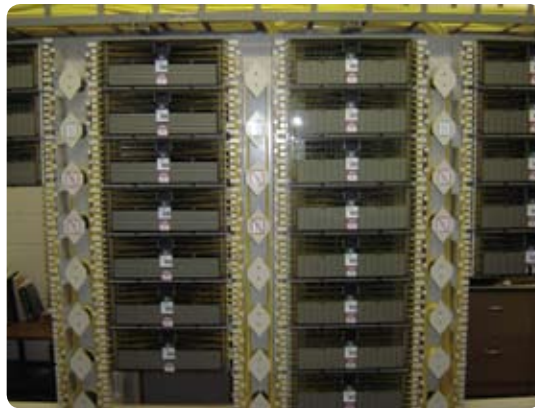
West Plains relies on ADC's Fiber Distribution Frame (FDF) panels and frames and FiberGuide® System to manage the current and expected volume of fiber in their central offices.
